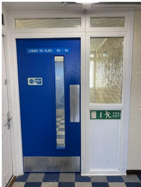
Communal Fire door set
