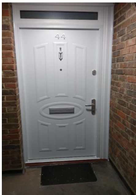
Front Entrance Fire door set
